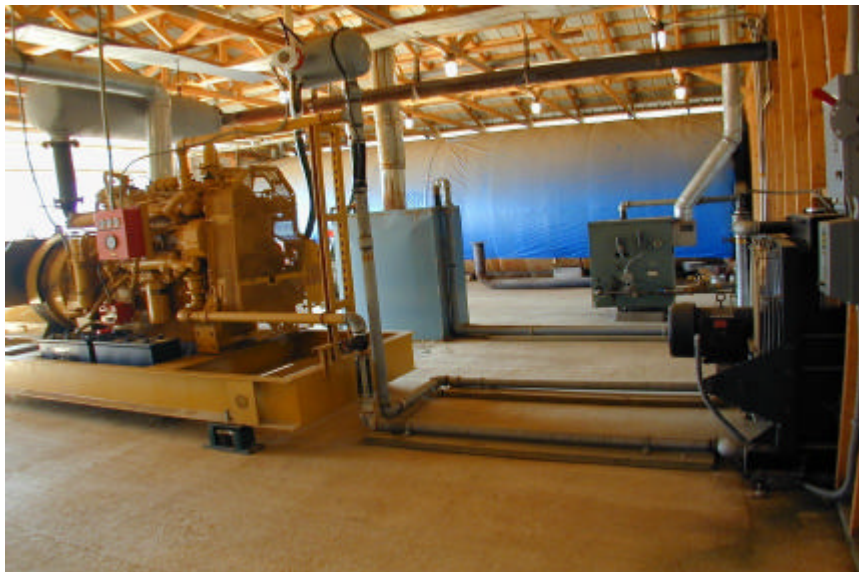
Figure 3. Barham Farms Biogas Combined Heat and Power
